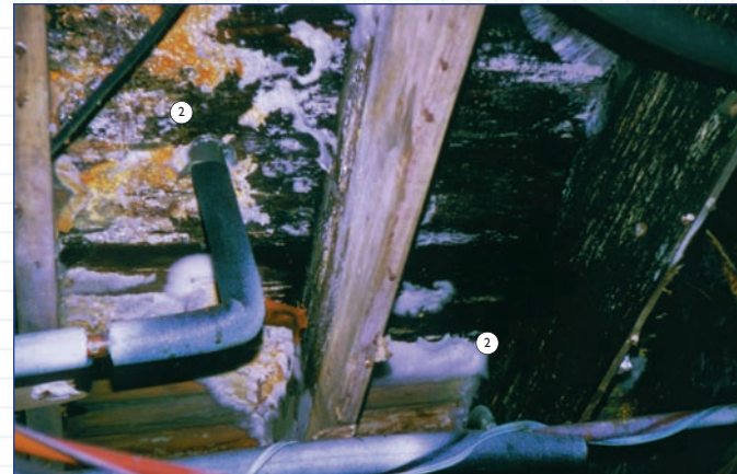
2) Various types of mold and mildew underneath the floors prior to remediation and installation of Icynene®
