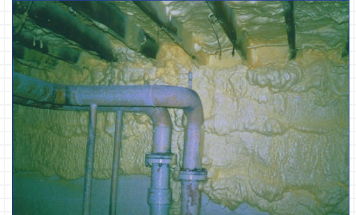
The gaps/cracks were sealed with Icynene® to prevent air leakage and from the above grade exterior.
