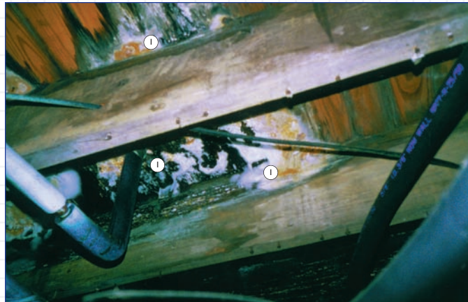
1) Mold problem underneath the floor prior to remediation and installation of Icynene®
